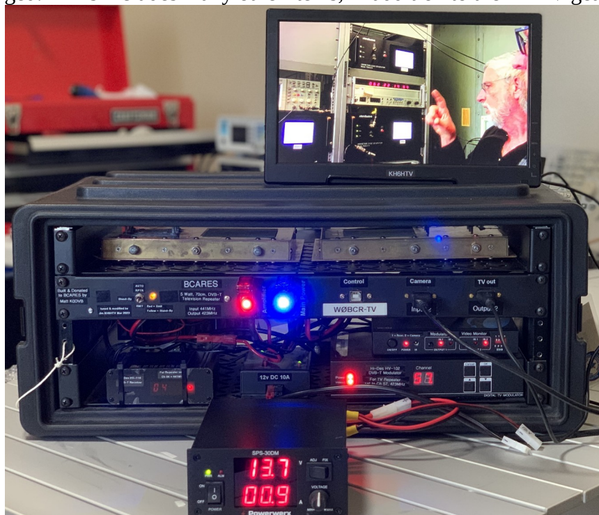
Matt's 70cm, 5 Watt, DVB-T Repeater
