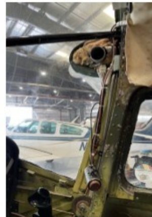
Coax and Control Cable Run
