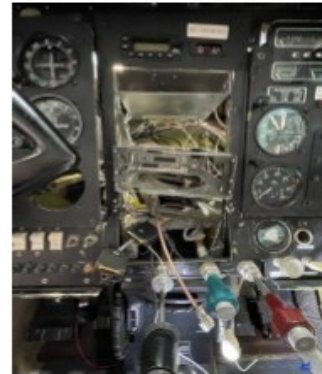
Center Stack opened up
