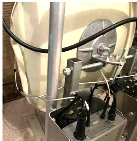
↑ Side damage to the microwave dish
