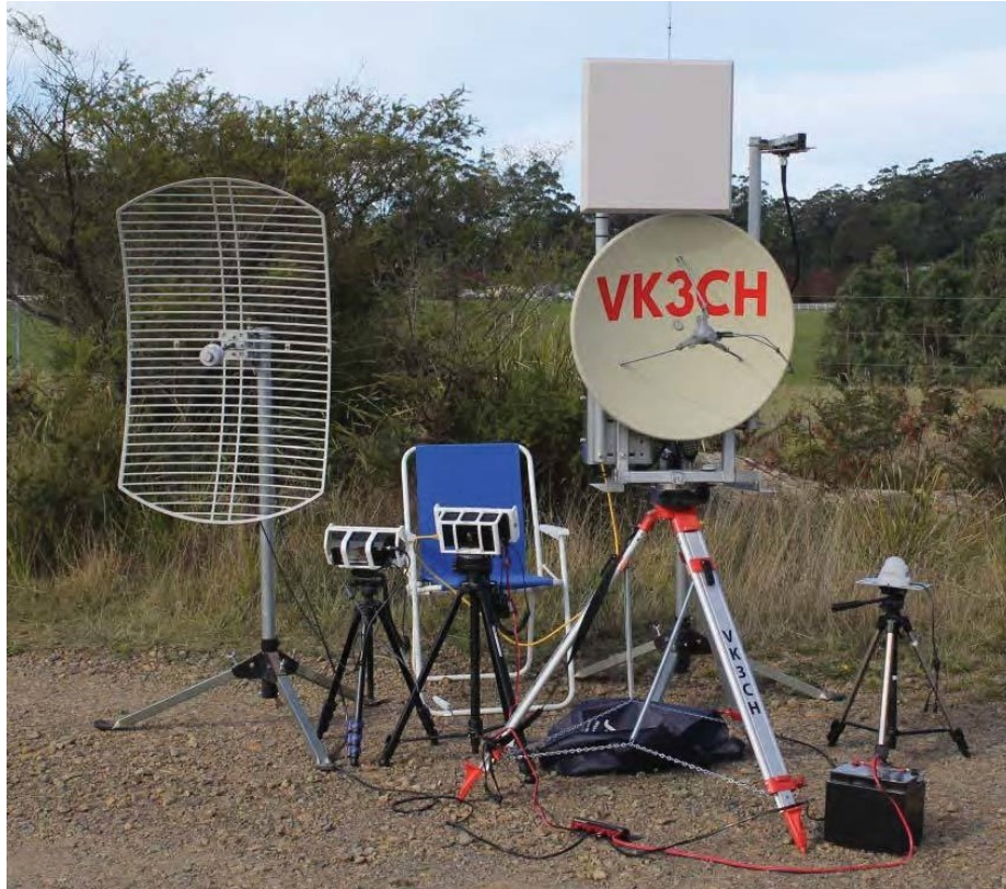
Photo of Mick's microwave antennas and gear taken on a calm day. Photo from his www.qrz.com web site.
